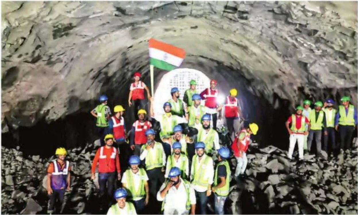
The 2.7-km stretch of the BKC-Shilphata corridor is located in Ghansoli, 400 metres away from Parsik Hills. Courtesy: NHSRCL
